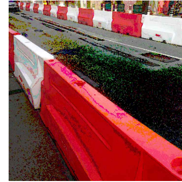
----- WATER FILLED ROAD SAFETY BARRIERS
